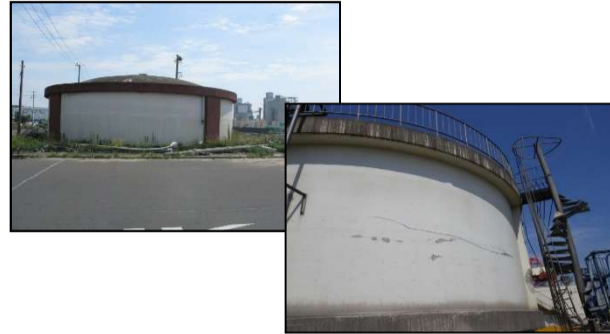
② PC tank affected by tsunami 1) L : Street lights and telephone poles collapsed, R : damages by a collision of overflow things
