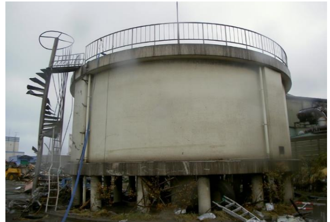
PC Tank that Withstood Tsunami
